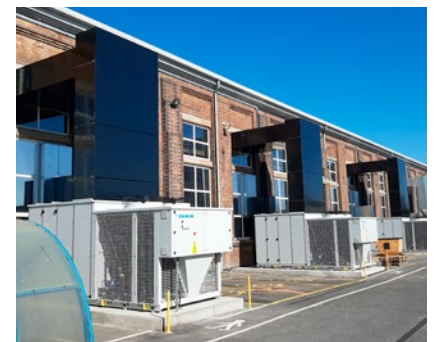
Air-to-air heating and cooling system, Paula Rosa Manhattan.
